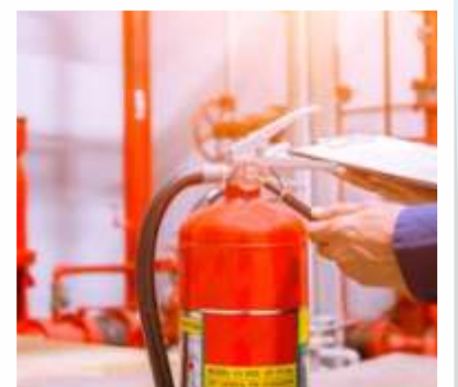
FIRE FIGHTING SYSTEM
